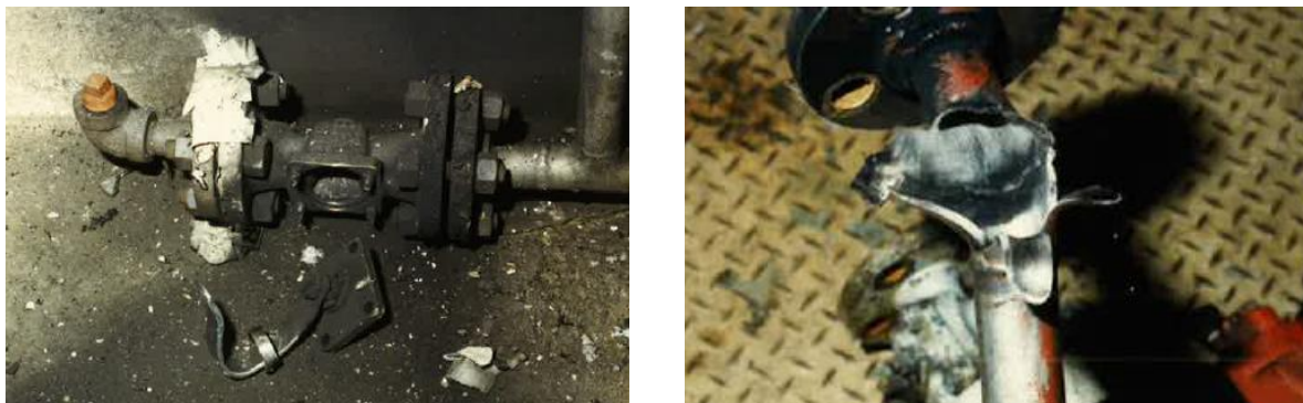
Figure 2 Damage from a TFE decomposition
